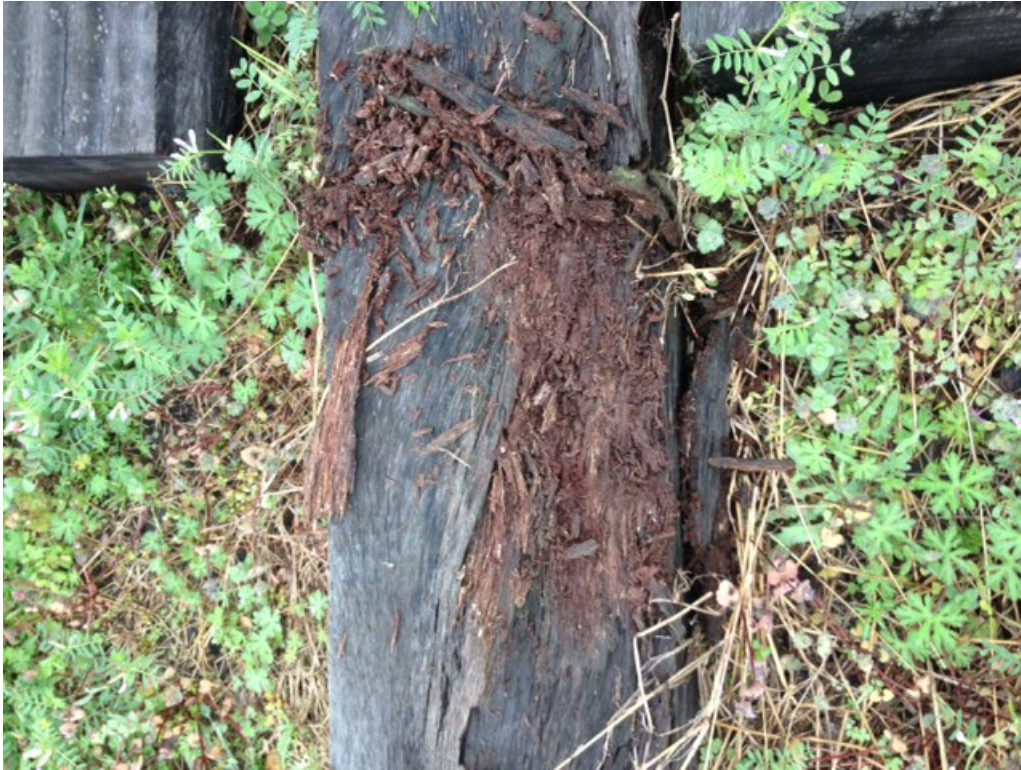
Figure 5 - Tie #9 (Turada) with decay.
