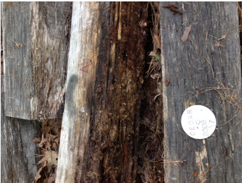
Figure 4 - Tie #4 bottom surface (white oak/control) with heavy decay.
