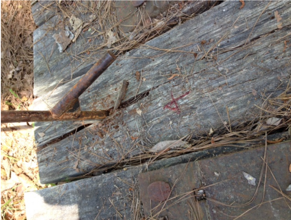
Figure 3 - Tie #4 (white oak/control) showing severe decay damage.
