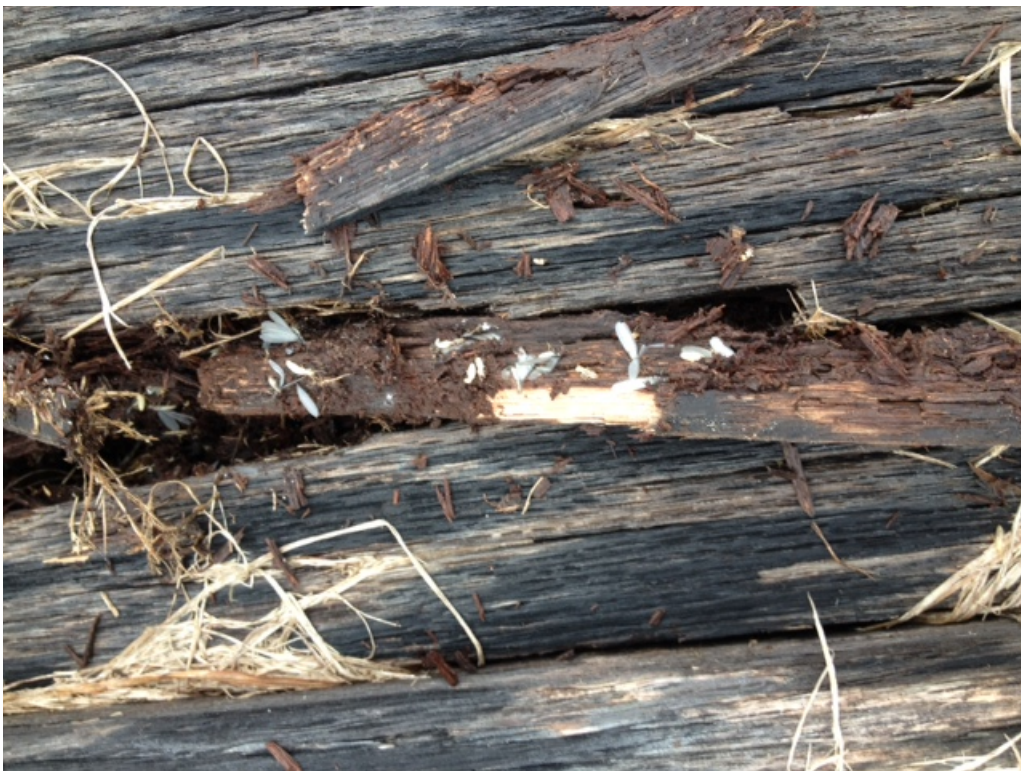
Figure 6 - Tie #209 with decay and termites present ( Reticulitermes ).
