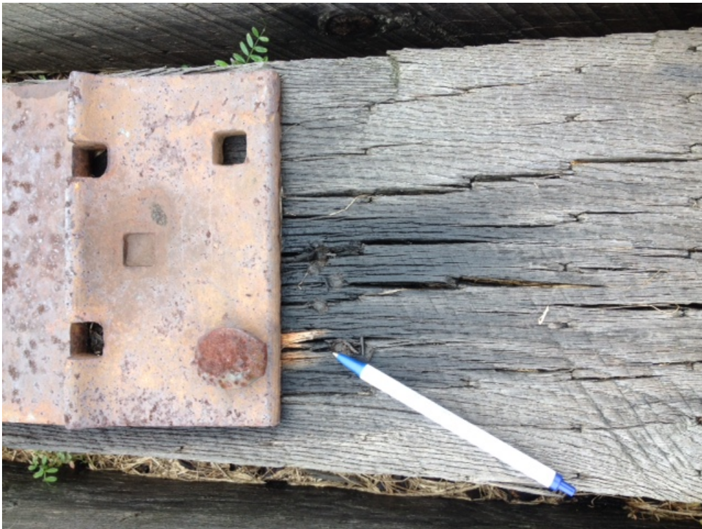
Figure 8 – Tie #223 with “iron sickness”.
