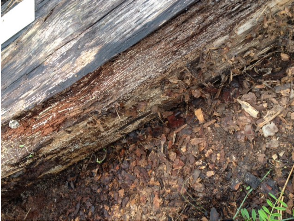
Figure 7 – Tie #83 with extensive decay.
